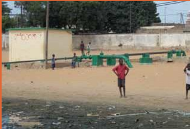
Groundwater pumping station in Dakar, Senegal
