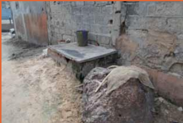
Domestic septic tank in Dakar, Senegal
