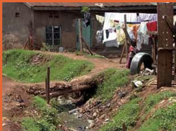
Poorly maintained drain channel in Kampala, Uganda
